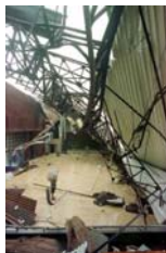
Fig. 2 Collapse of frame
