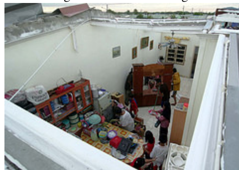
Figure 6f – Uplift Damage Roof Truss
