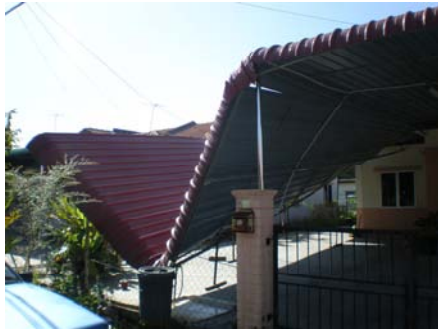
Figure 3a. Collapse Porch
