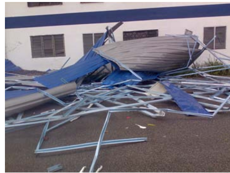
Figure 6b – Steel Truss failure
