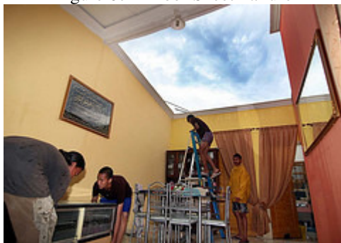
Figure 6e – Uplift Damage Roof
