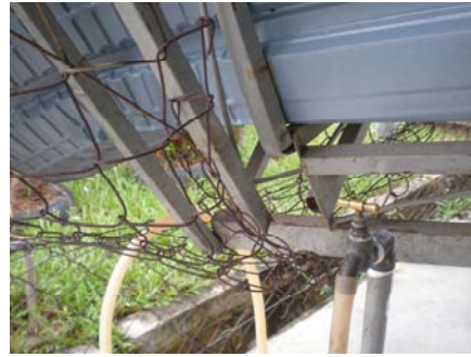
Figure 3b: Bending failure of Steel truss
