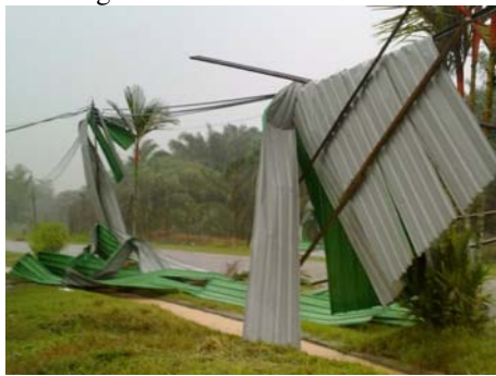
Figure 6c – Roof Sheet Failure
