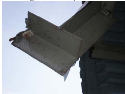
Figure 3c: Ultimate Load Failure
