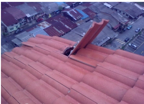
Figure 2a: Uplift Roof Tile
