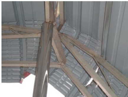
Figure 3d: Bending failure
