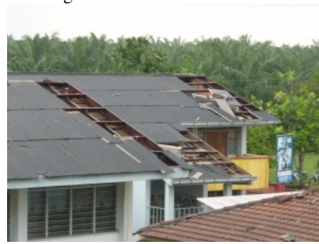
Figure 6d – Roof Damage
