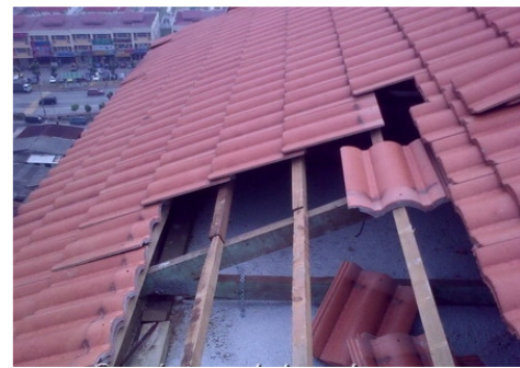
Figure 2b: Damage Roof Tile
