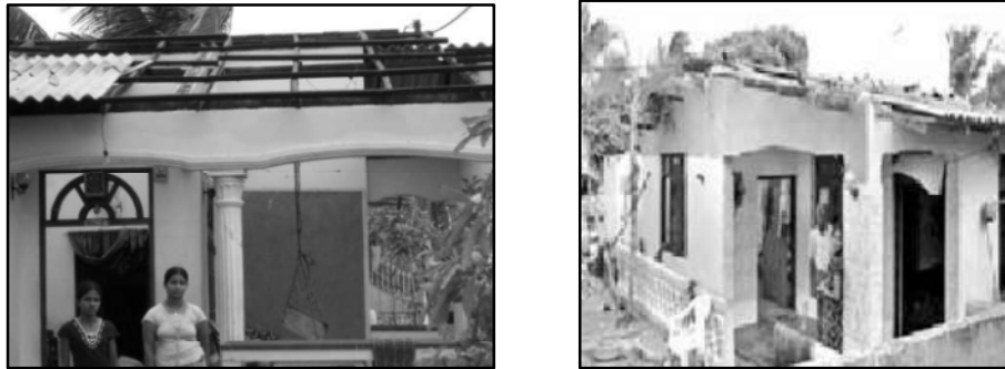
Figure 2. Damaged houses in Chilaw, Sri Lanka due to gale force on 16 th July 2009
